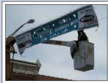
Installation of the new State Street Sign - 20th Annual Business & Consumer Expo Announcement
